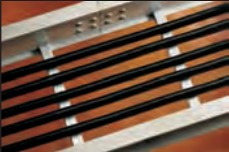
Instrumentation & Control Cables
