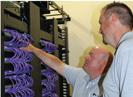
Built based on a mock TR evaluated during the IPD planning stages, Hallee (left) and Whitaker with E.S. Boulos deployed 1U blank panels above and below 48-port patch panels for each horizontal switch and used one-foot patch cords for aesthetics and manageability.
