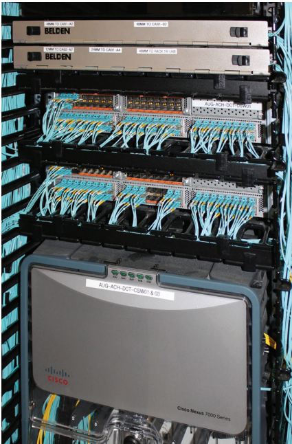
Designed using the latest switch fabric topology, the data center for MaineGeneral features two Cisco Nexus series 7010 core switches to distribute fiber to pods via Belden’s FiberExpress Ultra High-Density (UHD) rack-mount fiber connectivity system.
