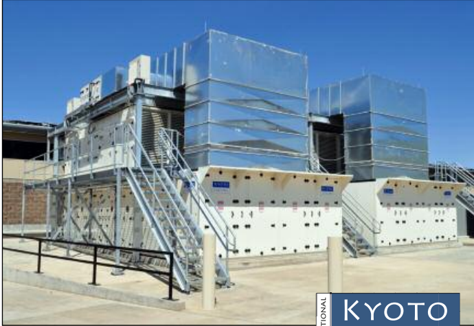
Two of the largest KyotoCooling® wheels in North America were installed at the Vault. Combined with CPI cabinets, they offer free cooling and a PUE as low as 1.2.
