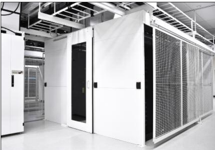
To create the flexibility and security needed in a colocation facility, the Vault implemented the use of performance optimized data centers, also known as PODs.
