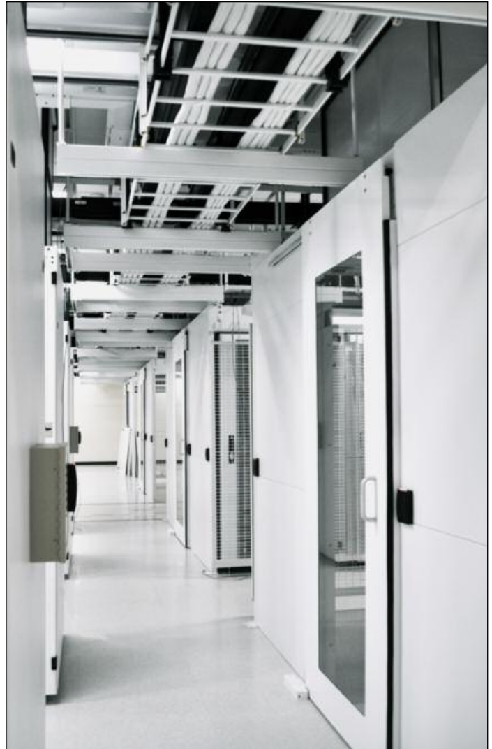
CPI used custom solutions such as white CPI Cable Runway and Cable Management to ensure the Vault’s aesthetics would match those of a display facility with a high tech appearance.
