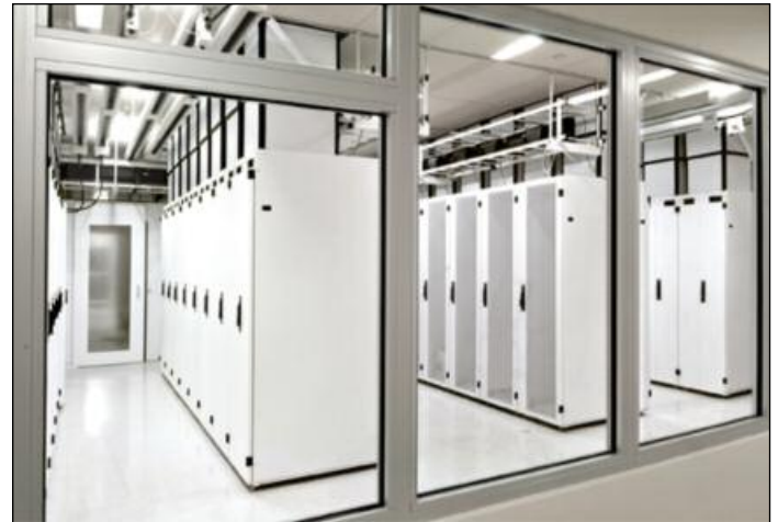
In an effort to build the greenest colocation facility in Oregon, the BendBroadband Vault deployed CPI Passive Cooling® and heat isolation by installing the F-Series TeraFrame® Cabinet System with Vertical Exhaust Ducts.
