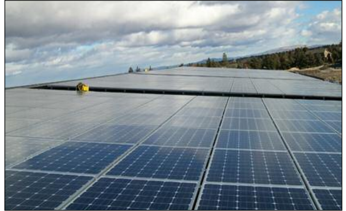
The Vault’s long list of green initiatives includes carbon credits, recycled building materials and the exclusive use of renewable energy from the local utility company, as well as a 152 kW solar array located on the facility’s roof.
