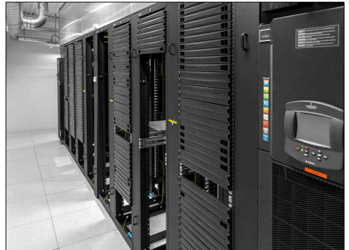
SpareBank 1’s state-of-the-art data centre gives them the flexibility to cool the equipment and maintain the continuity of operations.
