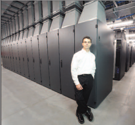
Eric Patterson, Data Center Manager for CDW played a strong role in the decision to install F-Series TeraFrame Cabinets equipped with CPI Passive Cooling Solutions in their new state-of-the-art data center.
