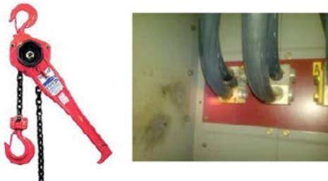
Figure 11 At left, a “come along” tool used for energized work and at right, damage to panel after phase to ground arc flash event with an upstream device with maintenance setting capabilities.
