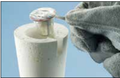
Fig. 9 Place the welding material cup into the top of the mold. Make sure the ignition strip nests into the recess on the top edge.
