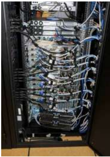
View of an enclosure using vertical patch and custom cable lengths
