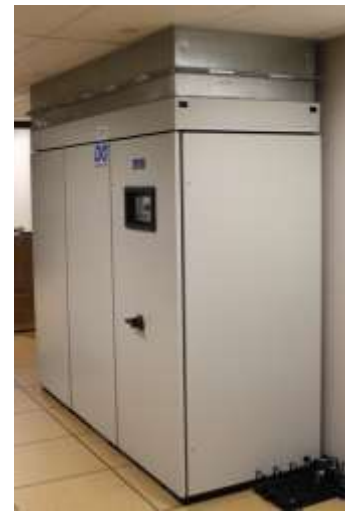
CRAC unit with plenum installed in the ceiling plenum for hot air intake
