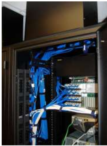
Cabling run from overhead to vertical patch installed toward the enclosure front which supports core switch
