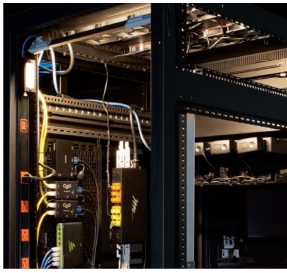
rackmount LED work light installed in the BGR rack
