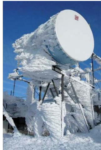
RFS Harsh Areas Line antennas help Pioneer Cellular maintain communications after a severe ice storm in Oklahoma, United States
