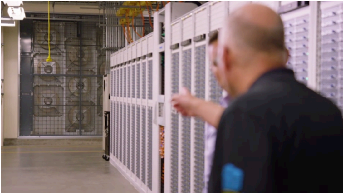
Figure 9- Fan wall inside Microsoft's fifth-generation data center in Quincy, Washington (Source: Microsoft video) 8
