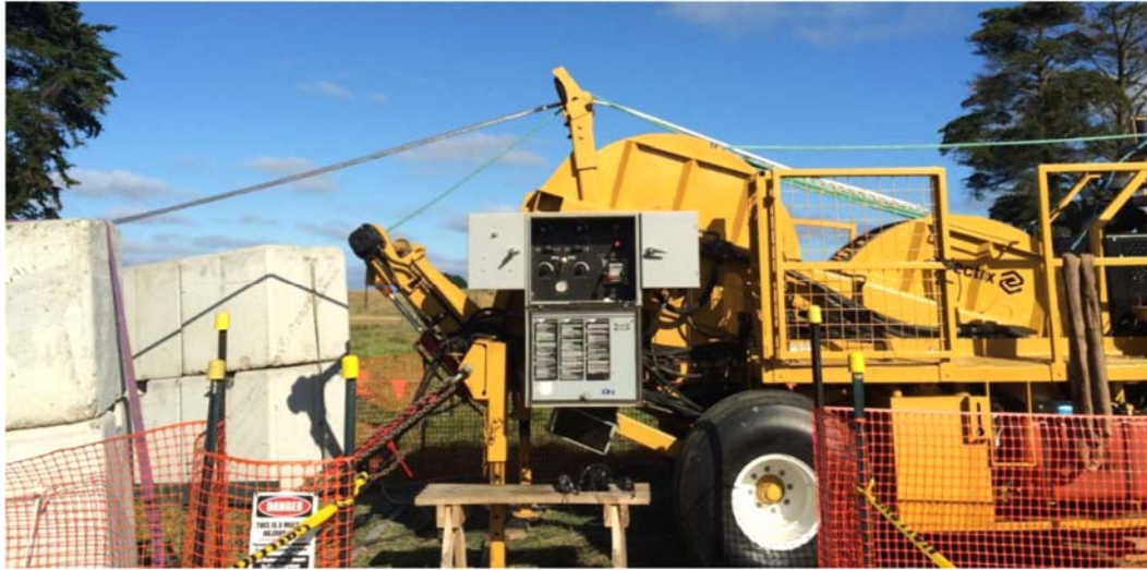
Figure 9. Adverse interaction of conductor with roller, courtesy of Transpower New Zealand.
