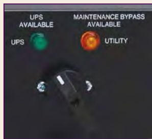
Maintenance Bypass Switch (Manual Transfer Switch)
