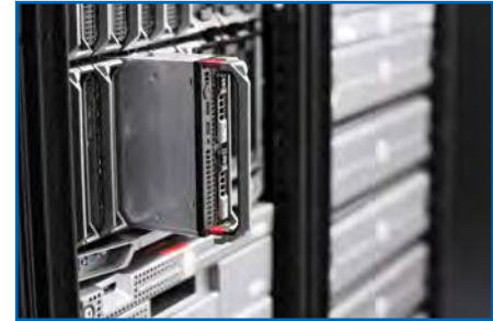
High-density loads like blade servers and PoE switches can create hot spots that traditional perimeter cooling systems have trouble addressing.
