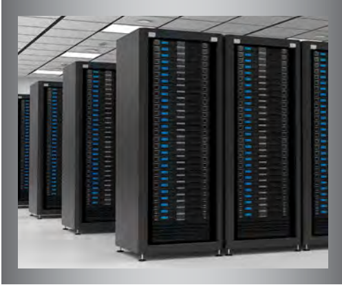
Your critical IT equipment requires around-the-clock protection.
