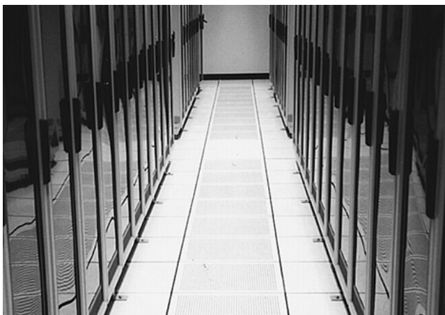
This cold aisle shows proper placement of perforated tiles on the intake side of IT equipment, but solid front doors may be impeding the intake of cooling air. This site may experience problems as product heat densities rise.
