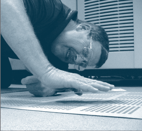
The troubleshooter card floating above the raised floor indicates an ideal airflow condition
