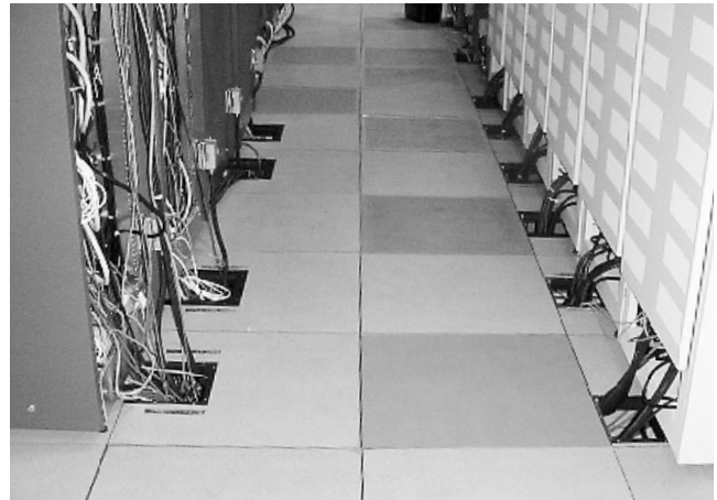
This hot aisle on the discharge side of IT equipment should literally be hot. Perforated tiles improperly placed in the hot aisle reduce cooling effectiveness.
