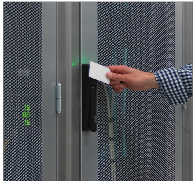
Real-time monitoring and managed access to server cabinet doors protect against malicious attacks or tampering.
