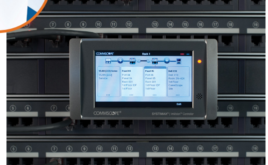
CommScope’s solutions support the next generation of data centres.
