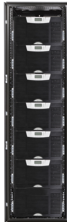
BladeUPS in a rack (60 kW, N+1 redundant)
