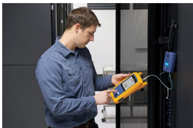
Accelerates data centre troubleshooting and certification
