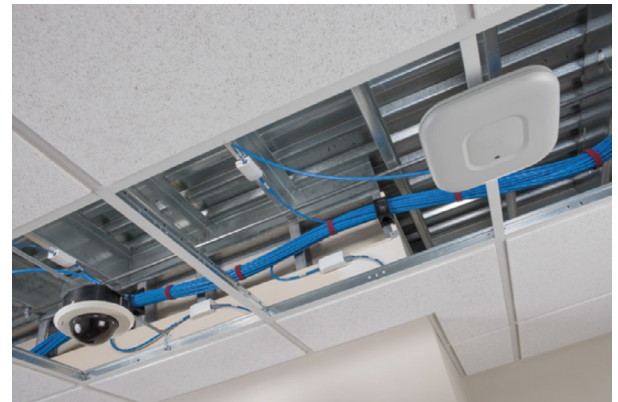
Category 6A cable is recommended for wireless access points and any devices that use Power over Ethernet.
