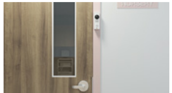
Network Video Door Station installed at entrance of nursery
