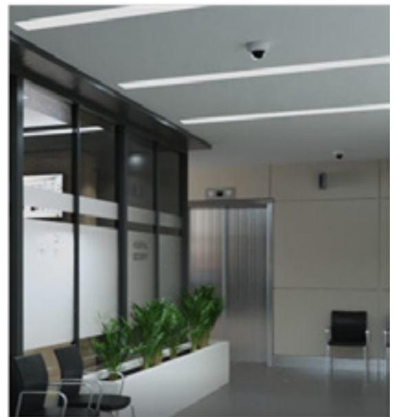
Axis P32s installed in hospital lobby
