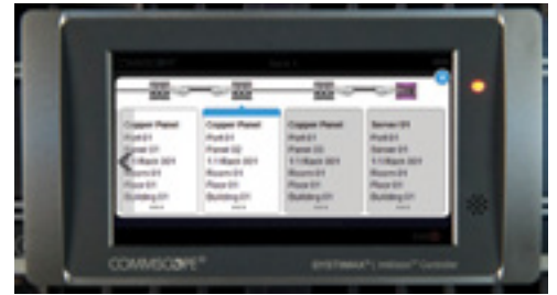
imVision controller showing circuit trace
