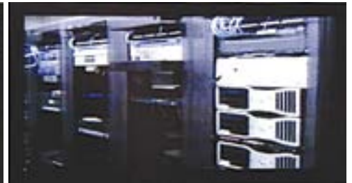
Using category 6A cabling
