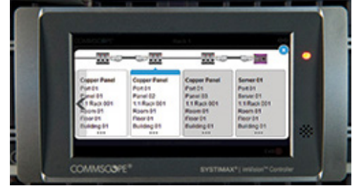
imVision controller showing circuit trace
